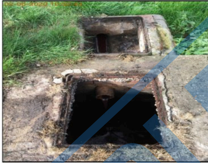
Photograph(s) of tank after the system was emptied:
